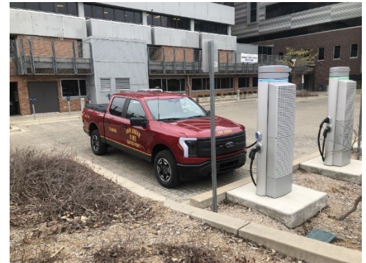
AAFD Electric Truck charging at City Hall.
